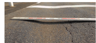
Fig. 2: Example of a road with surface distortion.
